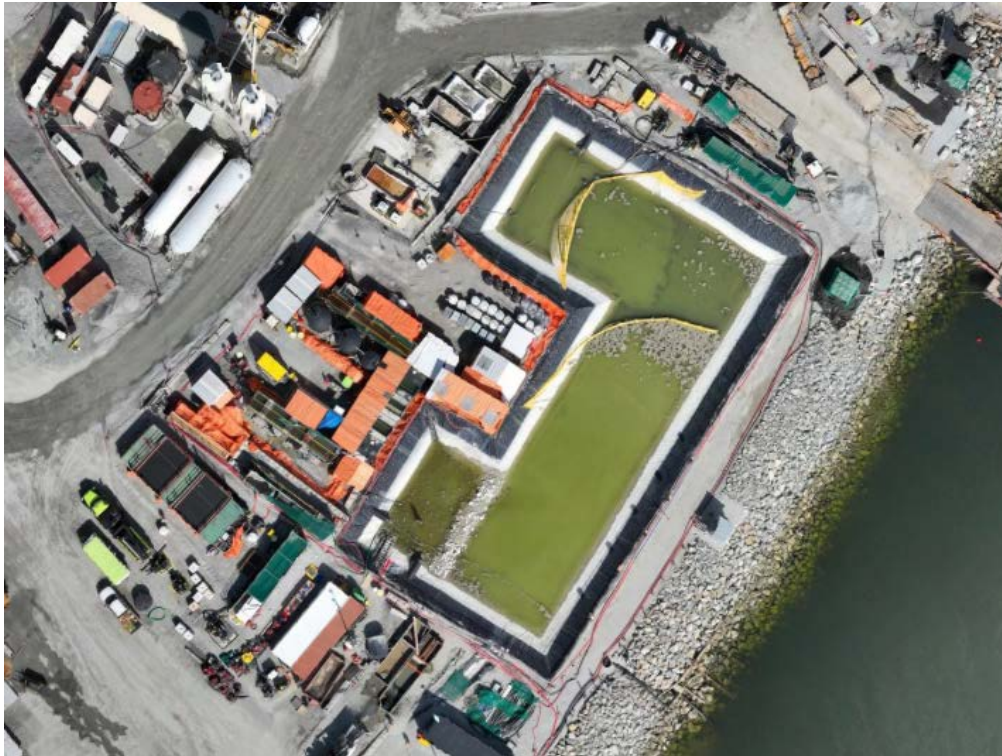
Figure 4: Aerial view of the East Sedimentation Pond (April 10, 2026). The East WWTP is located on the left side of the pond.
