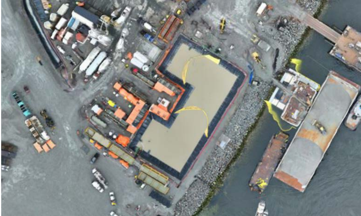
Figure 4: Aerial view of the East Sedimentation Pond (March 21, 2025). The East WWTP is located on the left side and the E500GPM TSS settling system is situated along the bottom edge of the pond.
