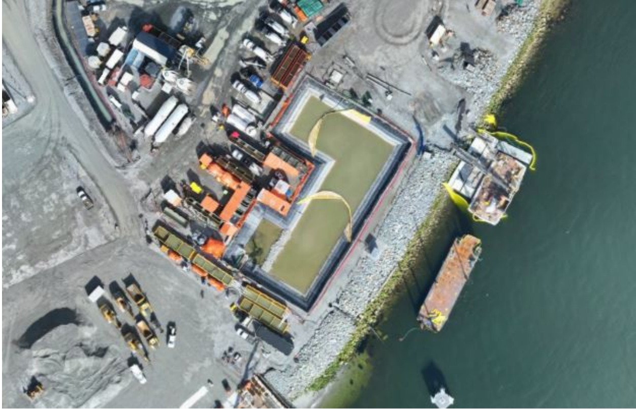
Figure 4: Aerial view of the East Sedimentation Pond (March 14, 2025). The East WWTP is located on the left side and the E500GPM TSS settling system is situated along the bottom edge of the pond.
