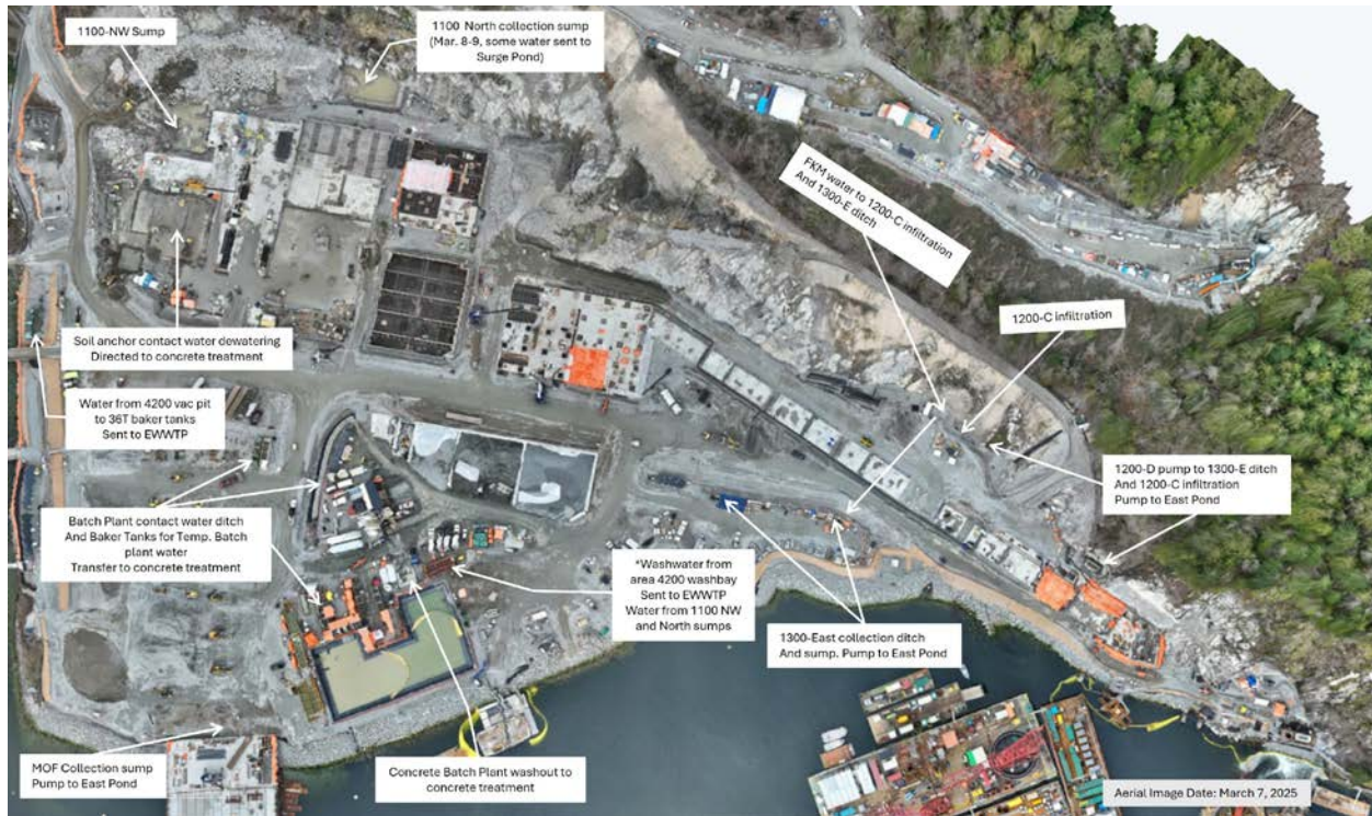
Figure 2: East Catchment contact water management facilities (March 9 – March 15).
