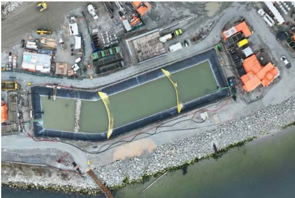
Figure 5: Aerial view of the West Sedimentation Pond (March 7, 2025). The TSS settling systems are located to the left (W500GPM) and right (ESC) of the pond.
