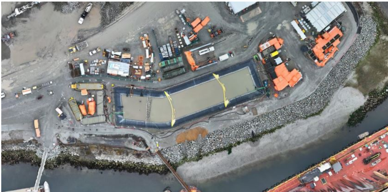
Figure 5: Aerial view of the West Sedimentation Pond (February 20, 2025). The TSS settling systems are located to the left (W500GPM) and right (ESC) of the pond.
