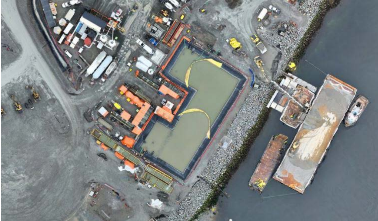
Figure 4: Aerial view of the East Sedimentation Pond (February 20, 2025). The East WWTP is located on the left side and the E500GPM TSS settling system is situated along the bottom edge of the pond.
