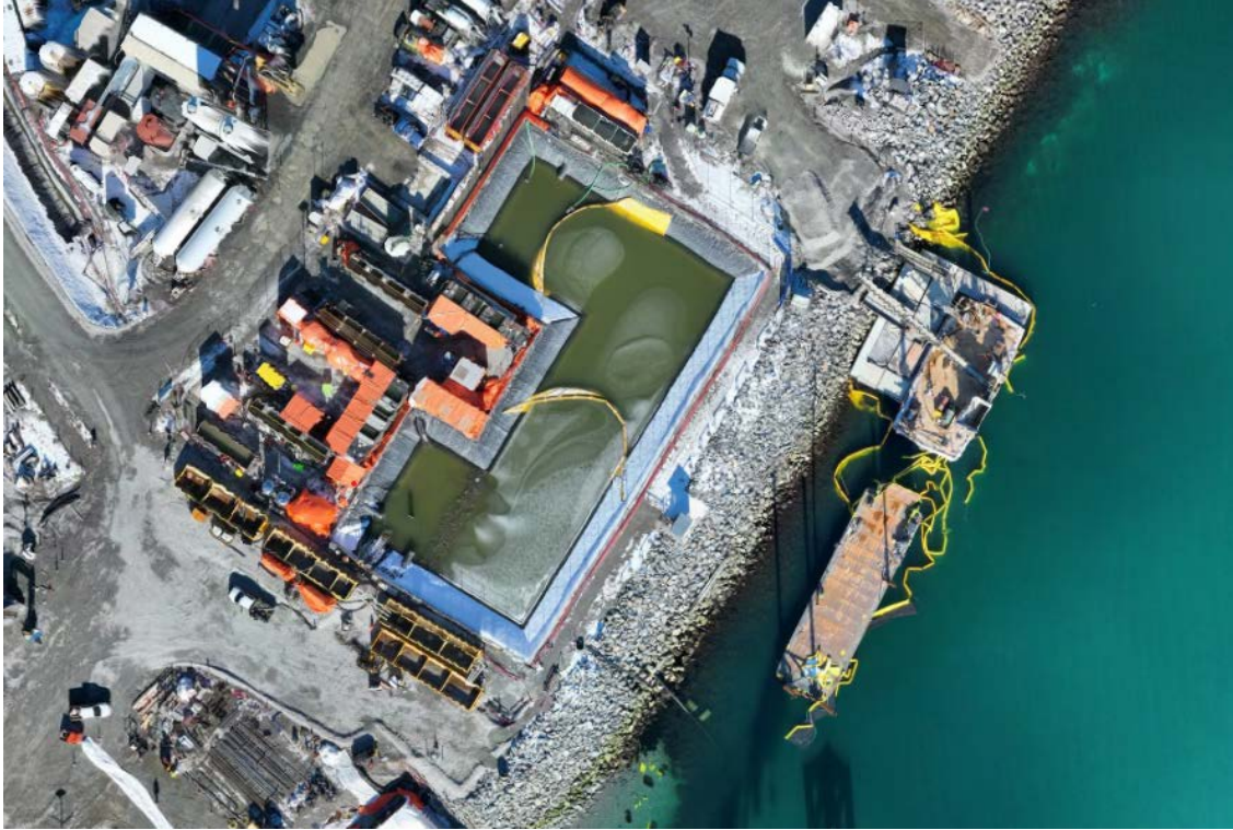
Figure 4: Aerial view of the East Sedimentation Pond (February 14, 2025). The East WWTP is located on the left side and the E500GPM TSS settling system is situated along the bottom edge of the pond.
