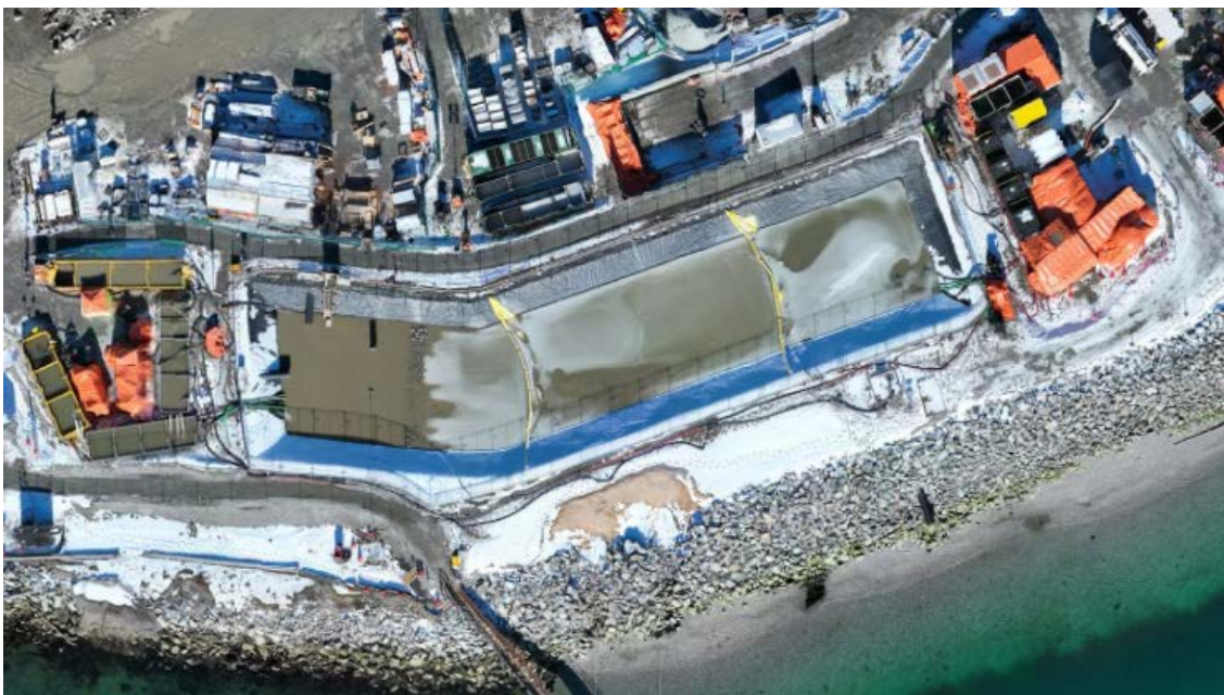
Figure 5: Aerial view of the West Sedimentation Pond (February 14, 2025). The TSS settling systems are located to the left (W500GPM) and right (ESC) of the pond.
