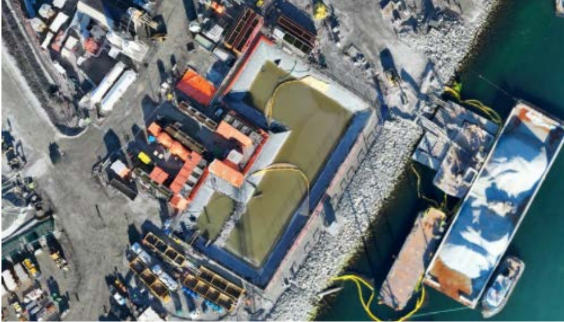
Figure 4: Aerial view of the East Sedimentation Pond (January 24, 2024). The East WWTP is located on the left side and the E500GPM TSS settling system is situated along the bottom edge of the pond.
