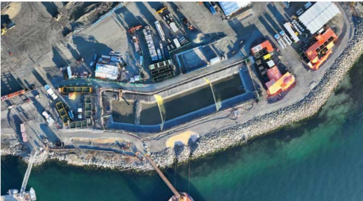
Figure 5: Aerial view of the West Sedimentation Pond (January 17, 2024). The TSS settling systems are located to the left (W500GPM) and right (ESC) of the pond.
