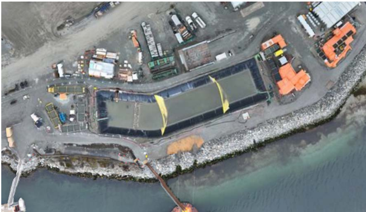
Figure 5: Aerial view of the West Sedimentation Pond (January 13, 2024). The TSS settling systems are located to the left (W500GPM) and right (ESC) of the pond.
