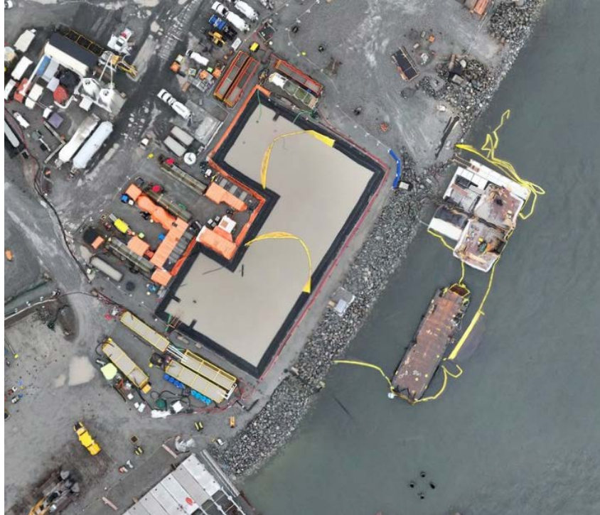
Figure 4: Aerial view of the East Sedimentation Pond (December 20, 2024). The East WWTP is located on the left side and the E500GPM TSS settling system is situated along the bottom edge of the pond.
