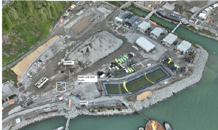
Figure 4 Details of the W LNG Onsite Daily Work (Construction) Activities for October 25, 2024.
