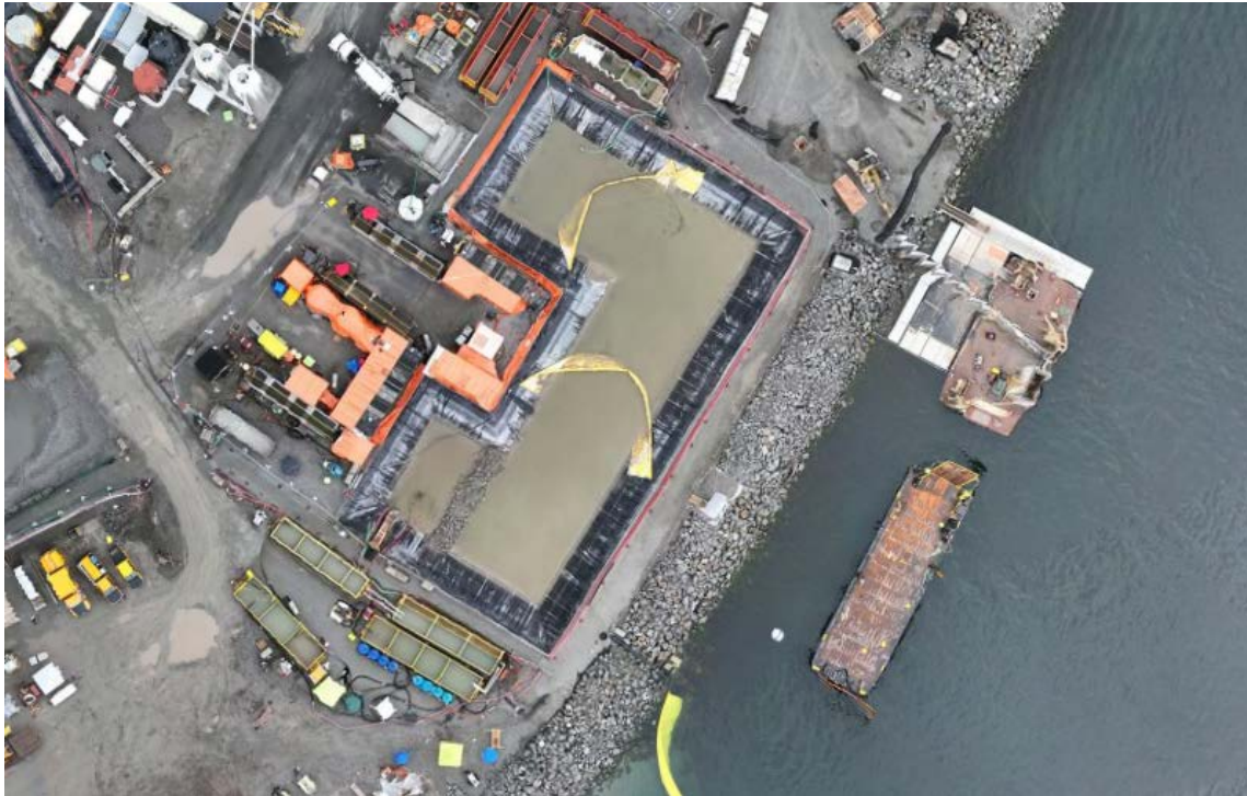
Figure 4: Aerial view of the East Sedimentation Pond (December 6, 2024). The East WWTP is located on the left side and the E500GPM TSS settling system is situated along the bottom edge of the pond.
