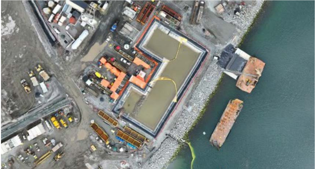
Figure 4: Aerial view of the East Sedimentation Pond (November 27, 2024). The East WWTP and the under construction East TSS settling (ESC) system are located on the left side of the pond.
