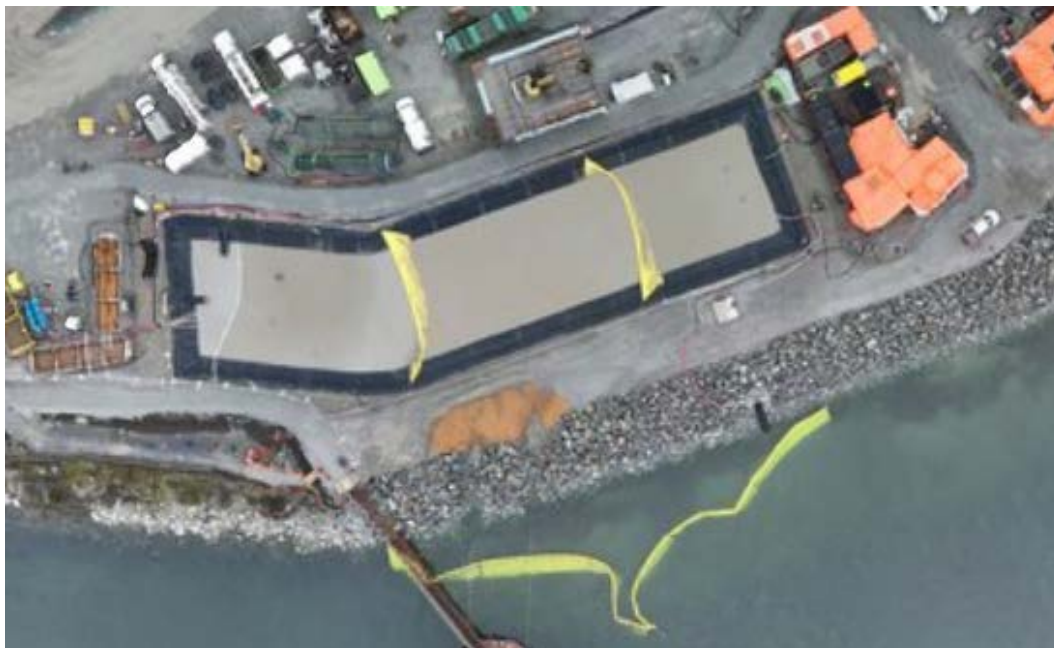
Figure 5: Aerial view of the West Sedimentation Pond (November 21, 2024). The TSS settling system (ESC System) and the West WWTP are located to the right of the pond.
