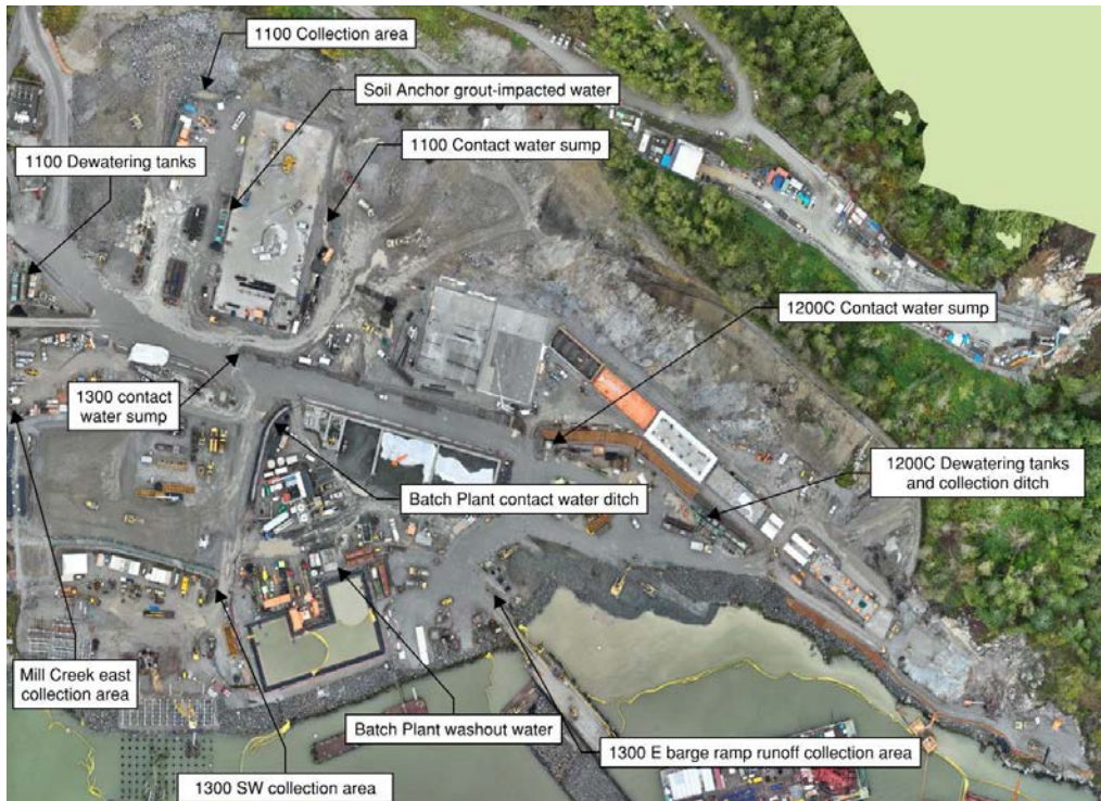
Figure 2: East Catchment contact water management facilities (November 10 – 16).
