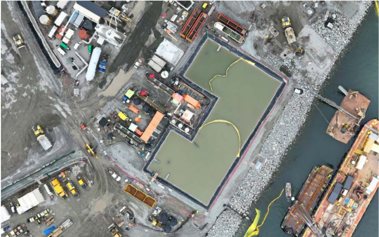
Figure 4: Aerial view of the East Sedimentation Pond (November 7, 2024). The East WWTP is located on the left side of the pond.
