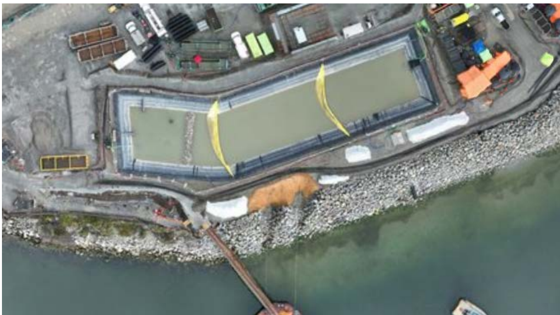
Figure 5: Aerial view of the West Sedimentation Pond showing the placement of two sediment curtains (November 2, 2024). The TSS settling system (ESC System) and the West WWTP are located to the right of the pond.
