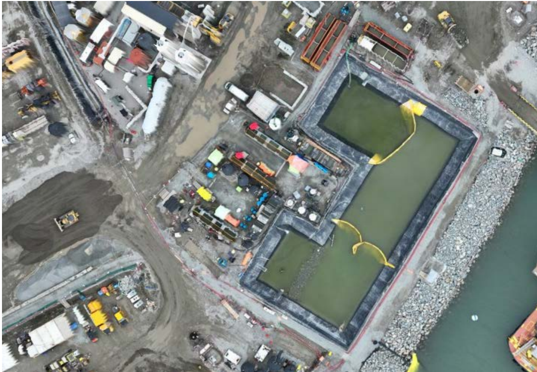
Figure 4: Aerial view of the East Sedimentation Pond showing the placement of two sediment curtains (October 25, 2024). The East WWTP is located on the left side of the pond.
