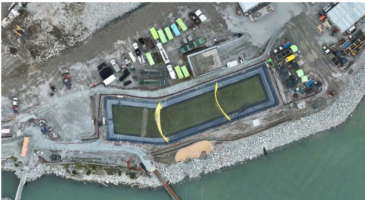
Figure 5: Aerial view of the West Sedimentation Pond showing the placement of two sediment curtains (October 25, 2024). The TSS settling system (ESC System) the West WWTP are located to the right of the pond.
