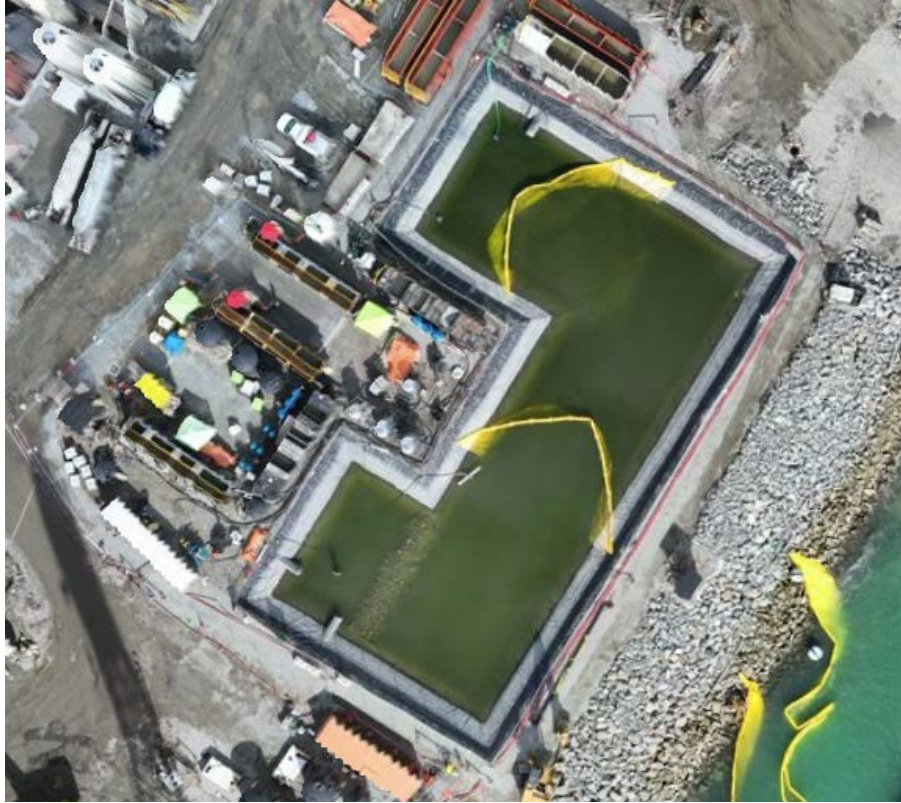
Figure 4: Aerial view of the East Sedimentation Pond showing the placement of two sediment curtains (October 2, 2024). The East WWTP is located on the left side of the pond.
