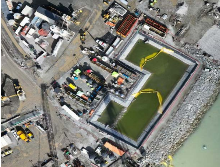
Figure 4: Aerial view of the East Sedimentation Pond showing the placement of two sediment curtains (September 27, 2024). The East WWTP is located on the left side of the pond.
