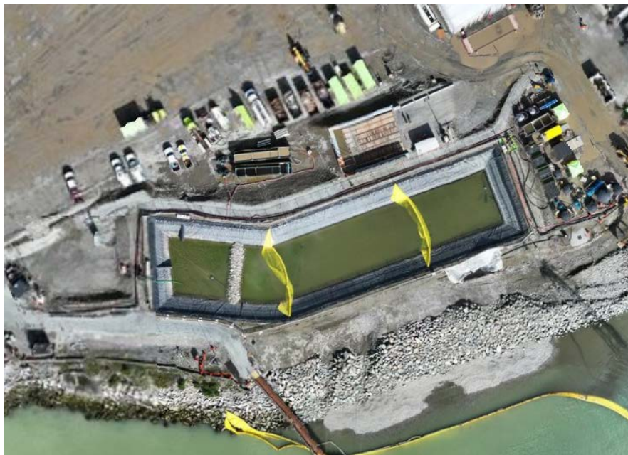
Figure 5: Aerial view of the West Sedimentation Pond showing the placement of two sediment curtains (September 27, 2024). The West WWTP is located on the right side of the pond.
