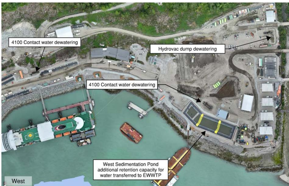
Figure 3: West Catchment dewatering areas. Dewatering of the West Catchment did not occur during the August 11 – 17, 2024 monitoring period.
