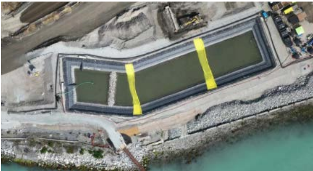
Figure 5: Aerial view of the West Sedimentation Pond showing the placement of two sediment curtains (August 9, 2024). The West WWTP is located on the right side of the pond.
