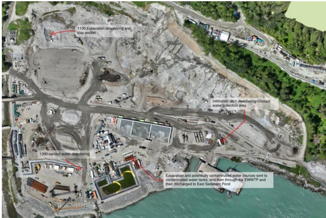
Figure 2: East Catchment Areas Dewatered to the East WWTP July 28 – August 3, 2024.
