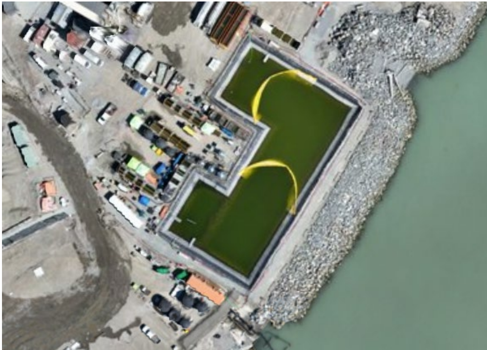
Figure 4: Aerial view of the East Sedimentation Pond showing the placement of two sediment curtains (July 12, 2024). The East WWTP is located on the left side of the pond.
