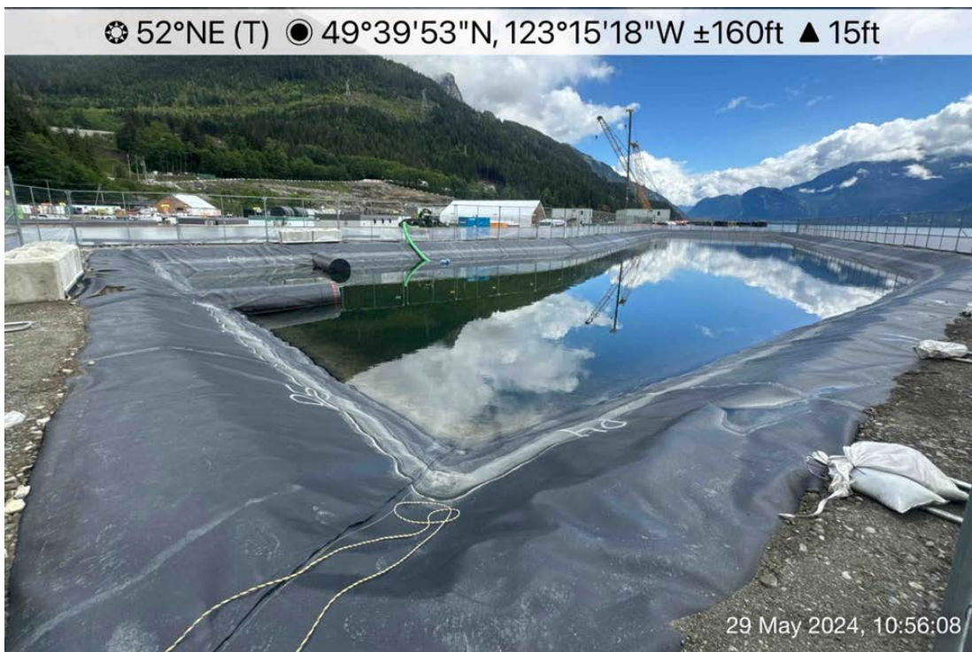
Figure 5: Ground level view of the West Sedimentation Pond, viewing northeast from the southwest corner of the Pond (May 29, 2024).
