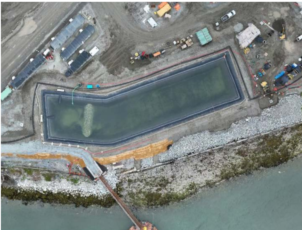
Figure 3: Aerial view of the West Sedimentation Pond and West WWTP (located west of pond) on May 25, 2024.
