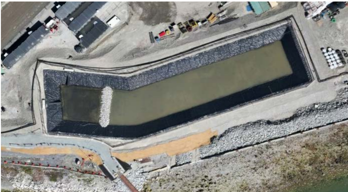
Figure 3: Areal view showing the current stage of construction for the West Sedimentation Pond and West WWTP (located west of pond) on May 10, 2024.
