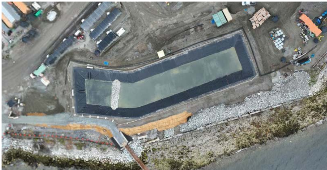
Figure 3: Areal view showing the current stage of construction for the West Sedimentation Pond and West WWTP (located west of pond) on April 25, 2024.
